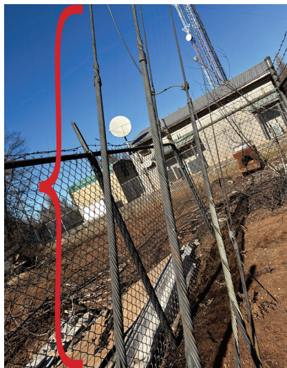
Fig. 2 — Photograph showing guy wires of anchor BB with visible discoloration.
