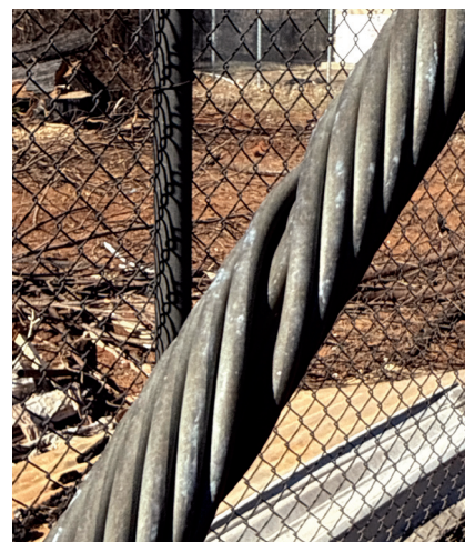
Fig. 4 — Closer view of one of the anchor BB guy wires clearly shows discoloration. Dark looking deposits are byproducts of combustion.
