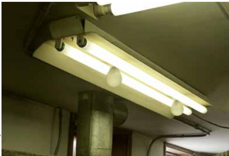
An incandescent/fluorescent hybrid: an early energy efficiency upgrade?
