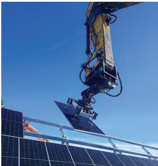
Diavik's new solar power plant is the largest off-grid solar facility in Canada's three territories.
