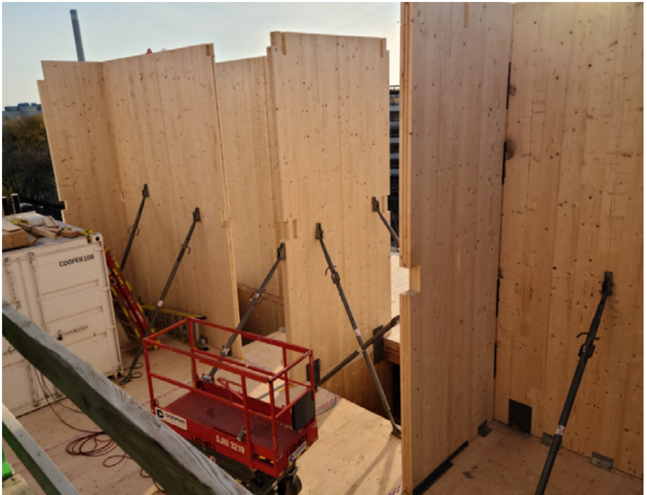
An all-wood mid-rise approach using CLT, replacing noncombustible materials. The exit stair enclosure is designed, built, and installed seamlessly with the structural assembly by using the alternative solution approach. PHOTO: Courtesy of Timber Systems Ltd.
