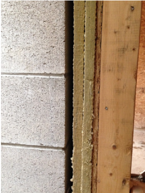
Isolation of the concrete masonry unit exit enclosure. Sound insulation is installed between the structural wood-framed wall and the exit stair shaft wall.
