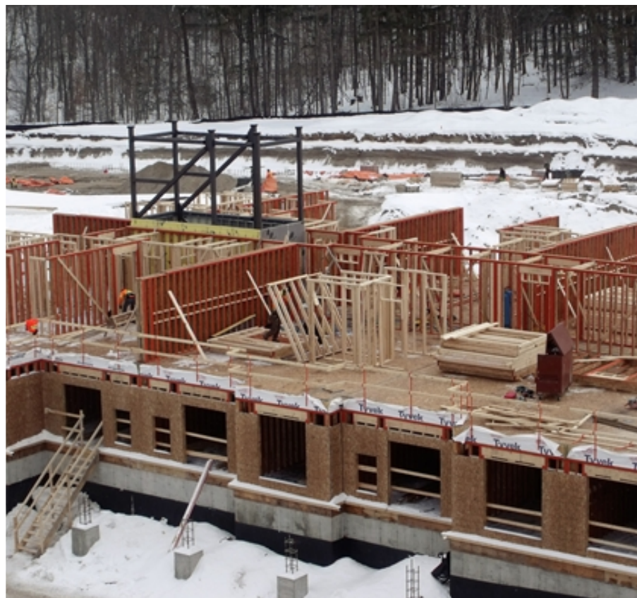
A steel shaft framing system being used for an exit stair enclosure.
