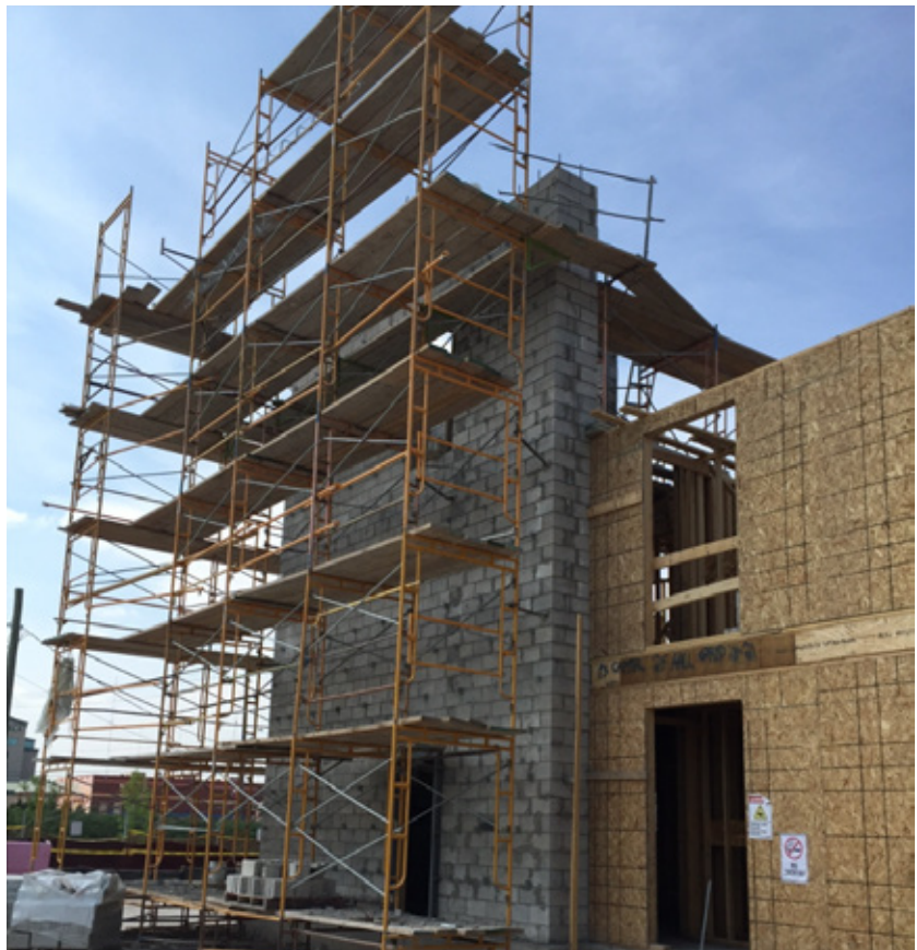
A noncombustible exit enclosure with wood-framed walls. Project management and coordination of trades become critical in maintaining build schedule.
