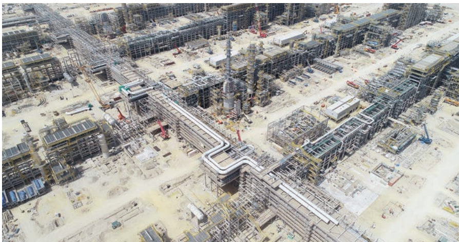
FIG. 2. Construction on the 615,000-bpd Al Zour refinery in Kuwait. The refinery was commissioned in 2Q 2022. Photo courtesy of Kuwait Integrated Petroleum Industries Co.
