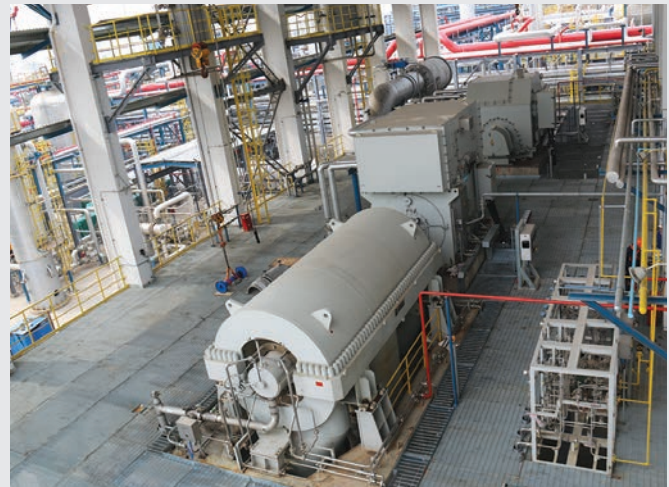
Elliott Centrifugal Compressor in Propane Dehydrogenation Service at a China Petrochemical Plant
