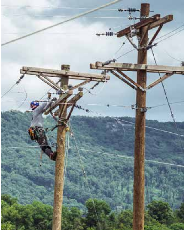
At Southeast Lineman Training Center, veterans can learn how to transition from the military into a well-paying career in the line trade.
